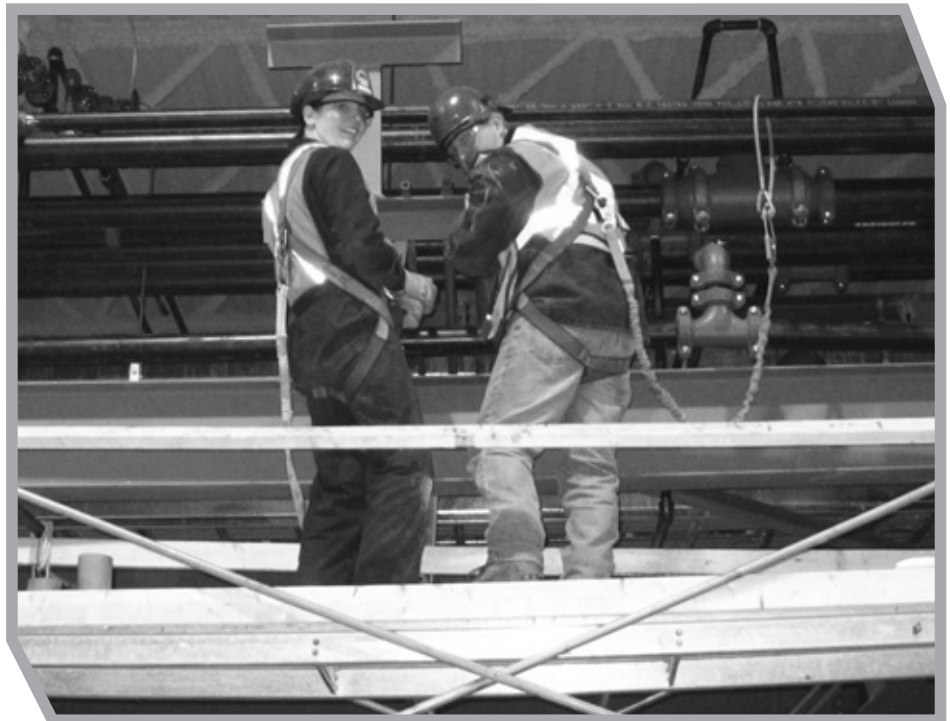
Maxine and John Cochrane are pipefitters working at the hydromet demonstration plant construction site
