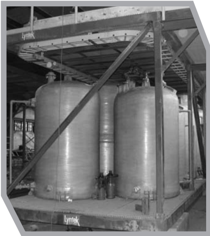
One of the process modules being assembled at Metal World's Argentia facility
