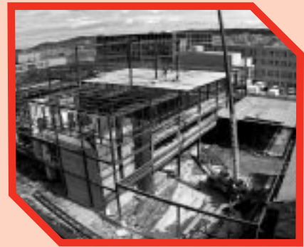
Construction activity at the Inco Innovation Centre (photo courtesy of MUN Photographic Services)
