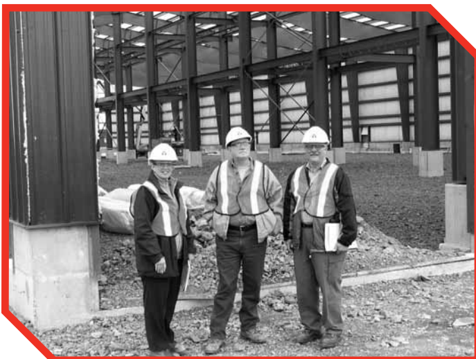
Environmental Health and Safety Audit Team at Argentia hydromet demonstration plant construction site
